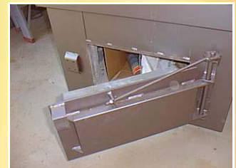
Ash Cleanout Door
